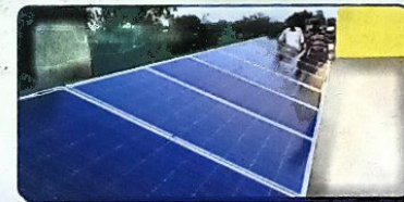
Solar Power Station
